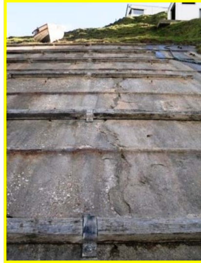
Concrete revetment – showing crack (Asset Ref No. 1221D901D1803C02)
