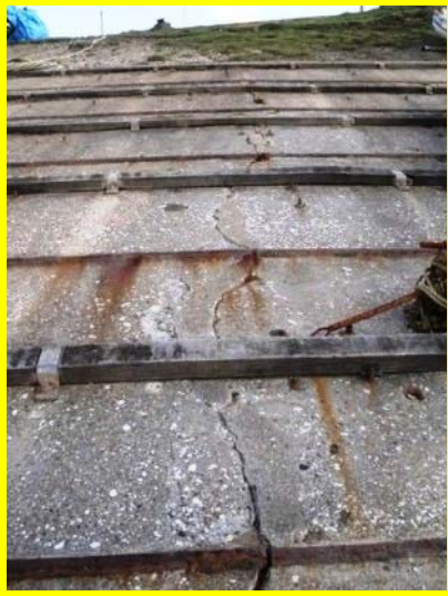
Concrete revetment – showing crack (Asset Ref No. 1221D901D1803C02)
