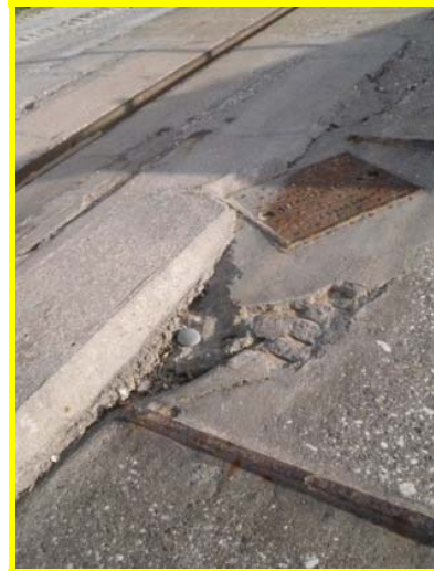
Failing repair around manhole (Asset Ref No. 1221D901D1803C02)
